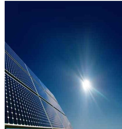
Vallelunga (Roma) 880 kWp plant Monocrystalline silicon
